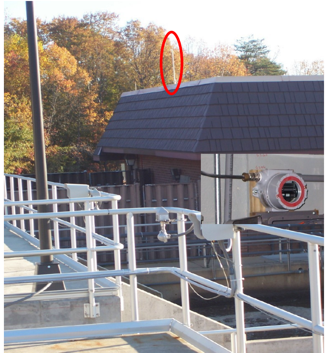
Base Radio Gateway mounted inside control room for ready access and integration with control system I/O
